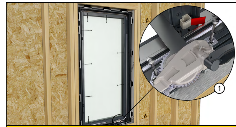
STEP 8 Shim and fasten at every installation hole and through the hardware base (1). Seal before fastening the sill.
