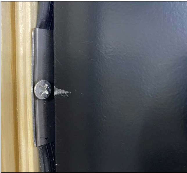
Figure 13 The cladding can be protected with nail fin or an extra bracket
